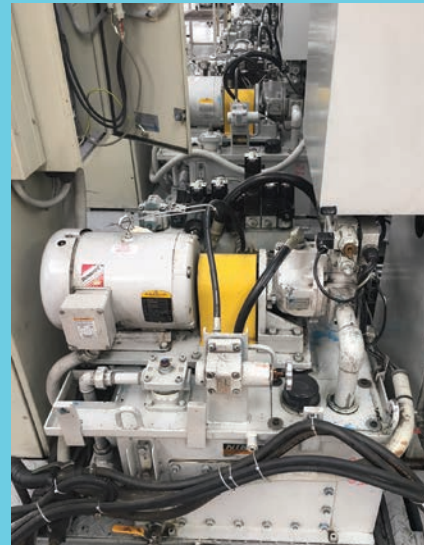
PREVIOUS MANUFACTURER UNIT
