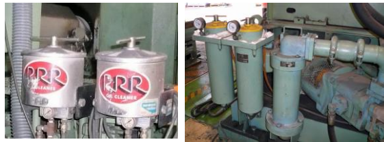
↓Company "R" Bypass filter & ↓Toshiba Off-line filter are unused(No exchange of line filters)
